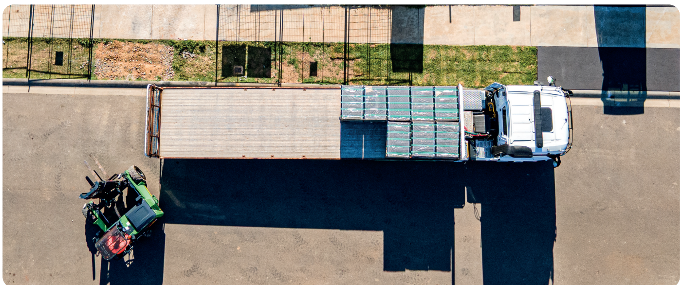
Greg Rogers in action, offloading bricks at a construction site with an all-electric MOFFETT E5 NX.
