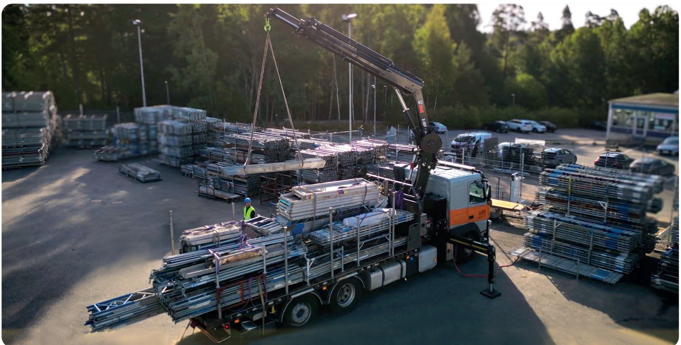
Kalle Björklund at work, loading a delivery of scaffolding with a HIAB X-HIPRO 302 crane powered by a HIAB wspir.
